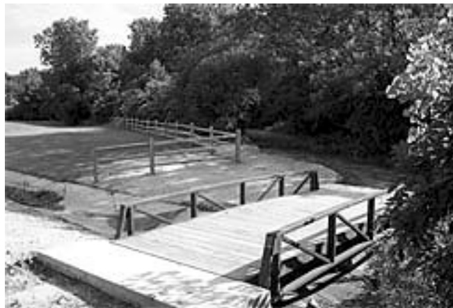
New trail and bridge under construction on the west campus of Midwestern University. Photo: G. Goodman.
