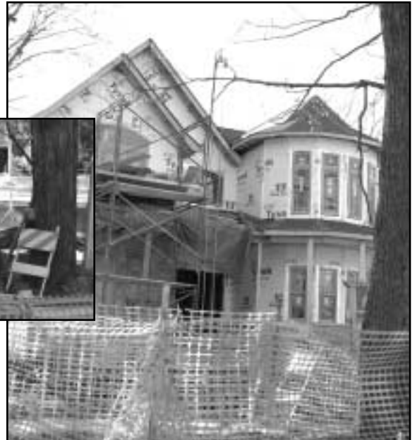
Construction damage causes significant damage to trees, which often do not survive.
